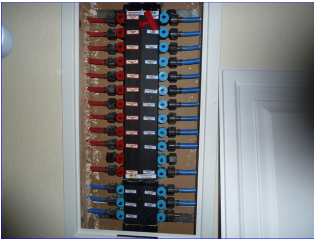
A. Item 2(Picture) PEX water system
