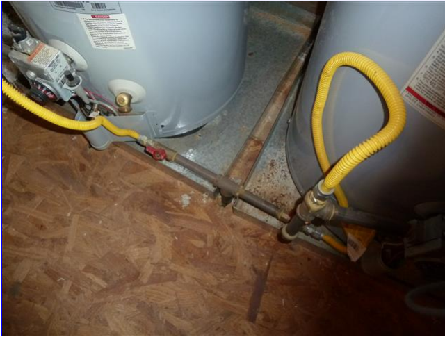
B. Item 1(Picture) No bonding between gas lines and water heaters.
