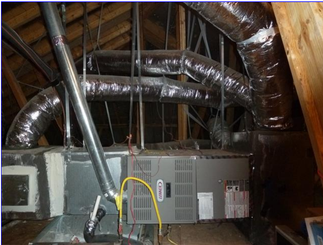
A. Item 1(Picture) Air handler/gas furnace
