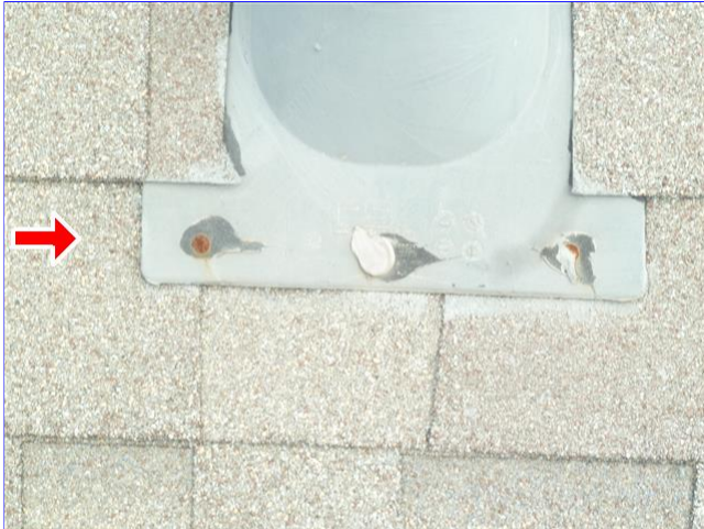
C. Item 1(Picture) Caulk over the exposed nail heads.
